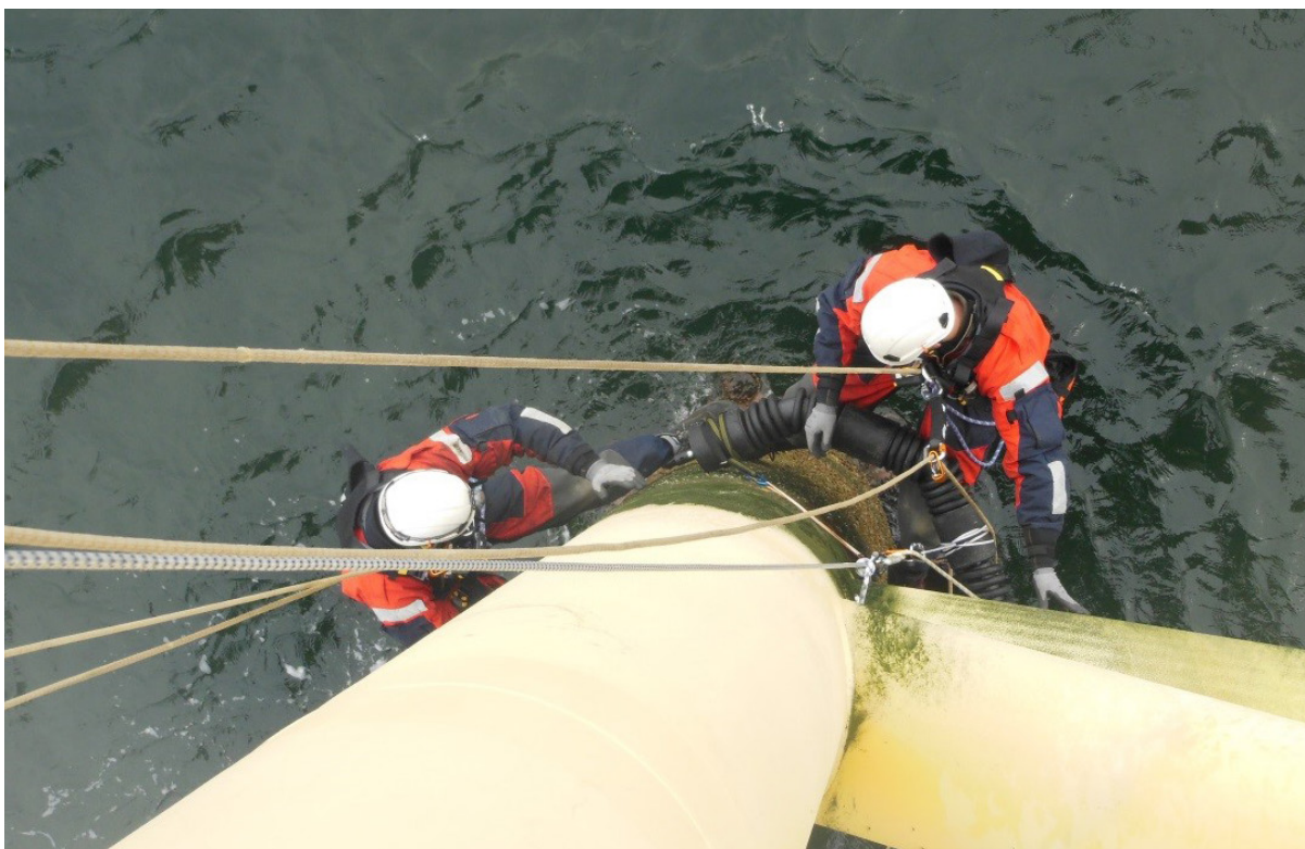
Figure 6: Fitting leg cleaning device to minimise marine growth buildup (photo reproduced with the permission of Found Ocean Ltd.)
