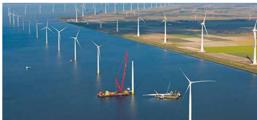
Figure 1. The last wind turbine being placed in Lake IJsselmeer at the Westermeerwind/Noordoostpolder wind farm
