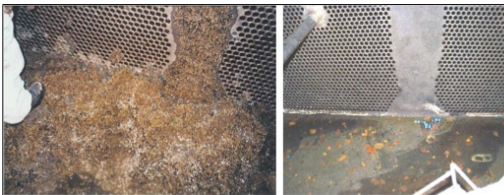
Figure 14. Pulse-Chlorination at the Maasvlakte Power Station, Rotterdam
