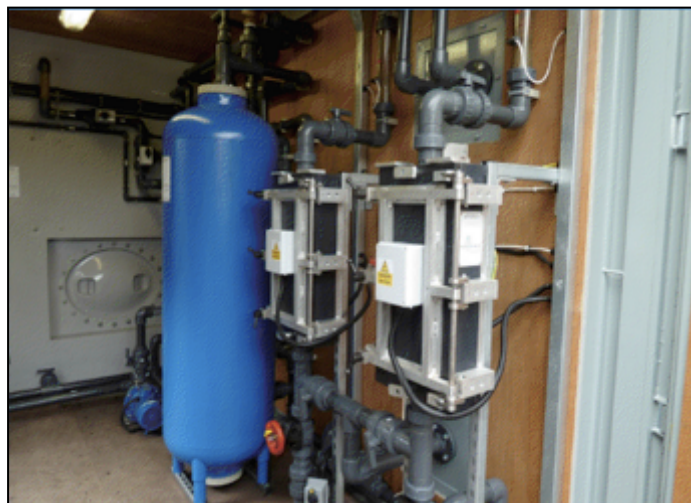
Figure 15. A Small Electrochlorination Plant on Board a Ship. Gulf Green Environmental, 2014
