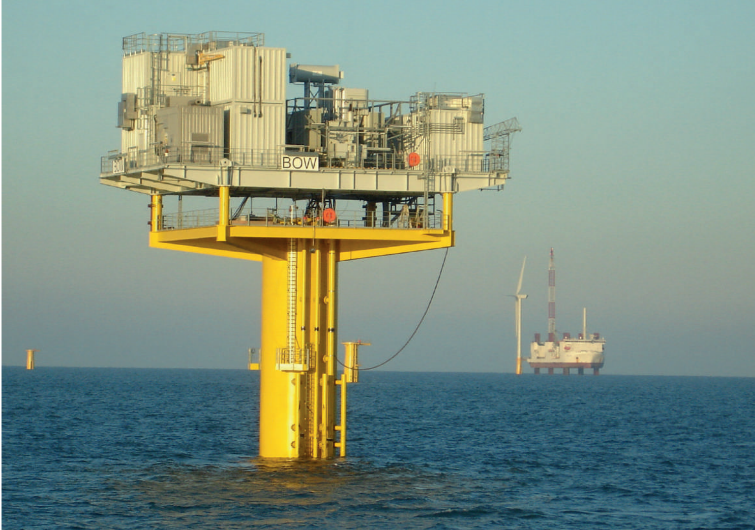
Figure 3. Offshore Substation (Source: Ramboll)
