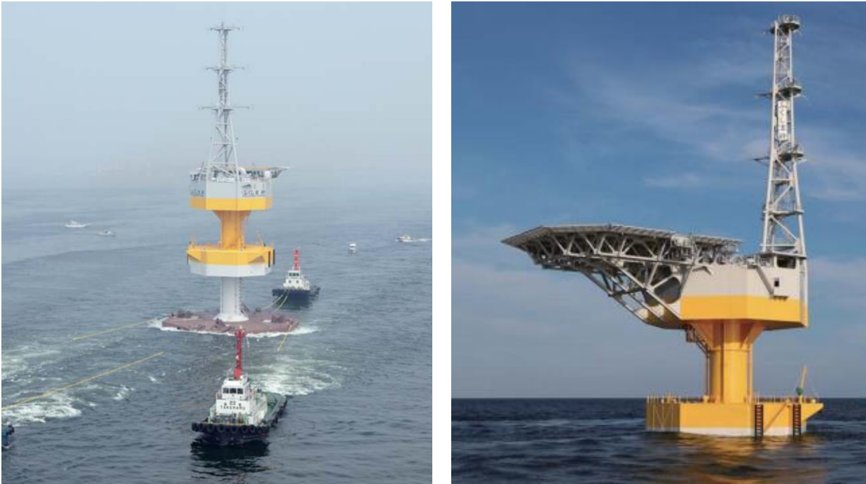
Figure 8: The 'Fukushima Kizuma' floating offshore demonstration substation project, rated at 25 MVA, (left) FOSS being towed out to site [11].
