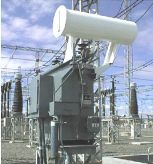
Figure 21 - Typical power transformer and conservator [98].
